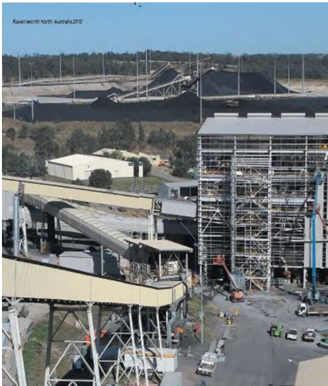
Spiral plant treating coal At Ravensworth North, NSW, using spirals specifically designed for upgrading coal fines
