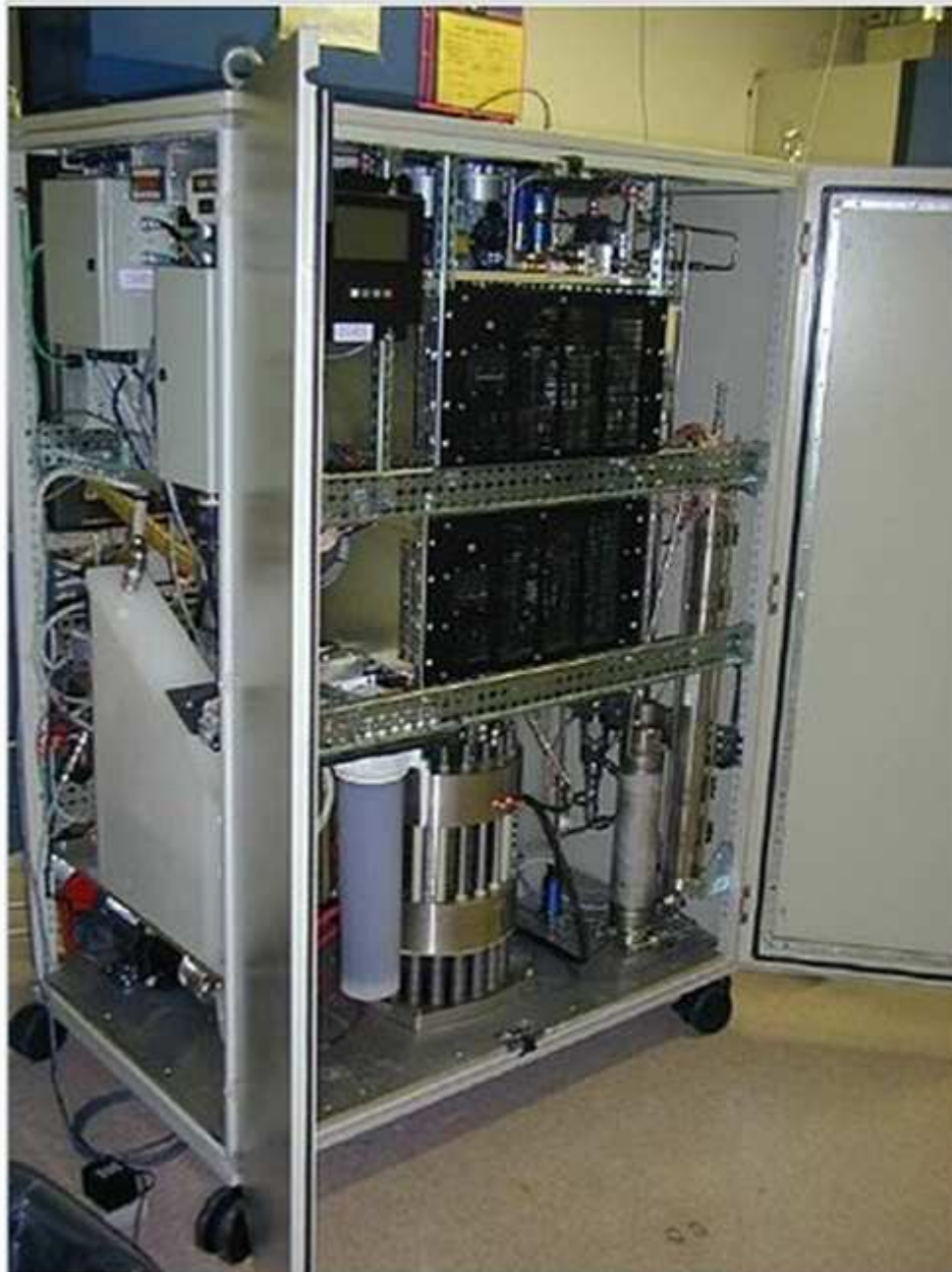
PEM high pressure electrolyzer system
